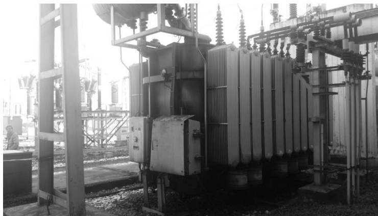
SLIKA 2 – ENERGETSKI TRANSFORMATOR MINEL TPv-7504-31.5
